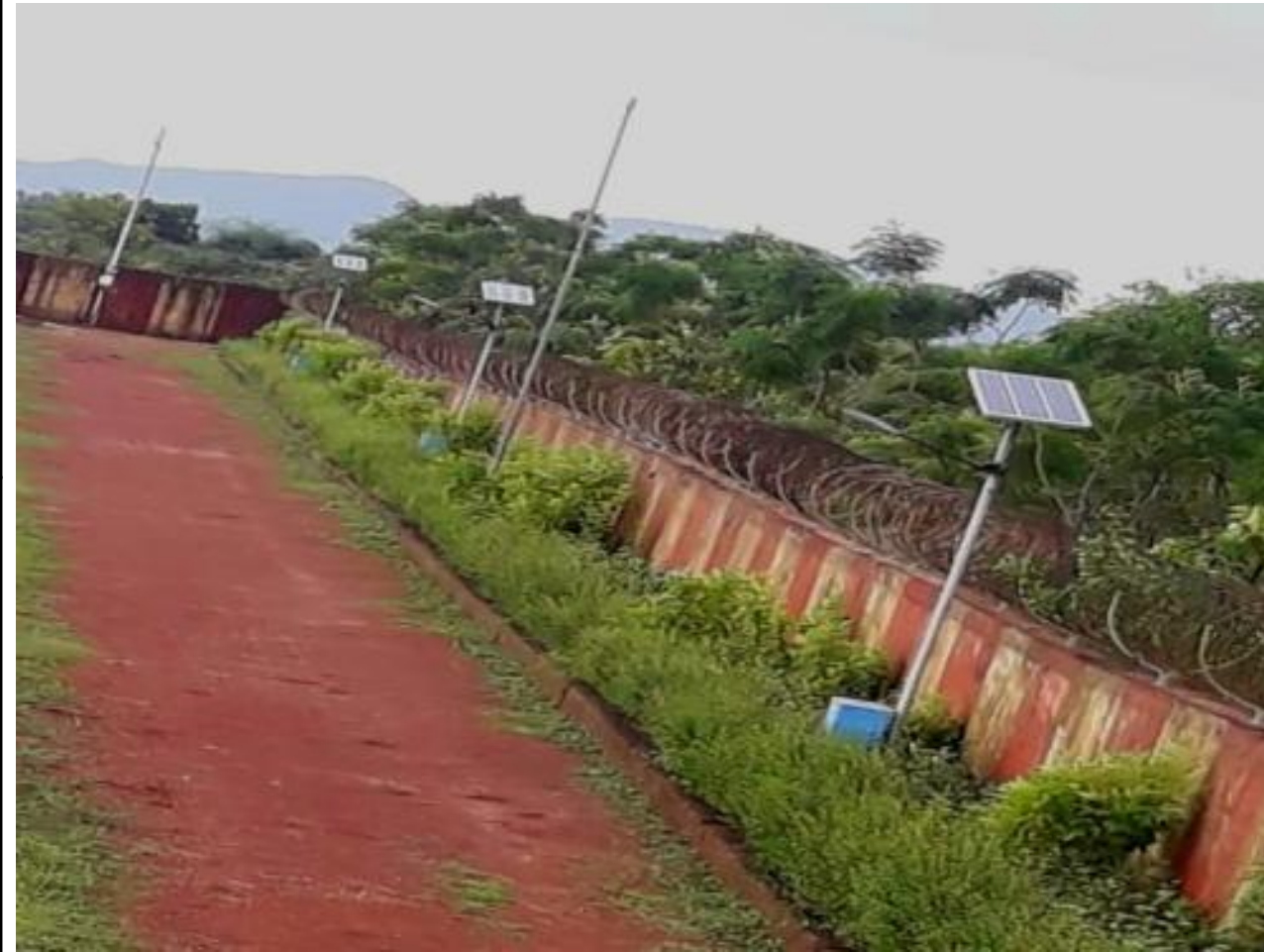
Installation of 125 no.s 50watt Solar Street light for plant area lighting and main road lighting
