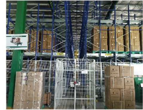
AUTOMATED STORAGE & RETRIEVAL SYSTEM
