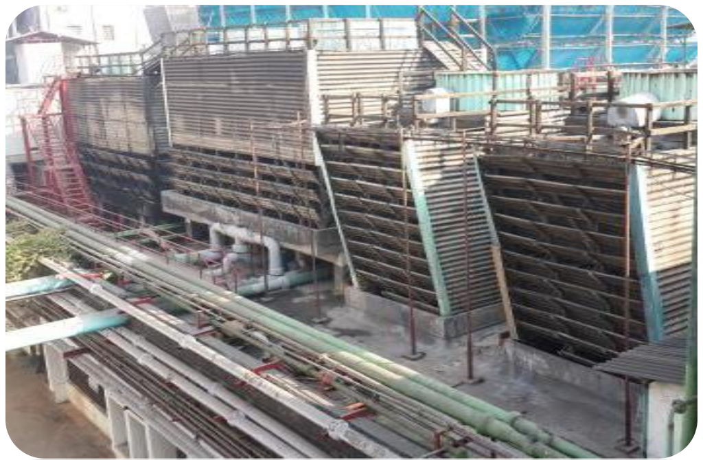
Old Cooling tower Power Consumption -168 KW
