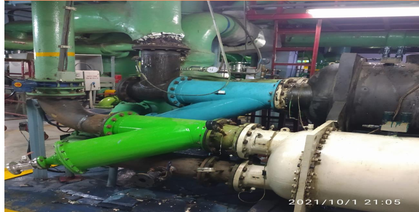
After Modification (Ball Cleaning System in Condenser & Evaporator)
