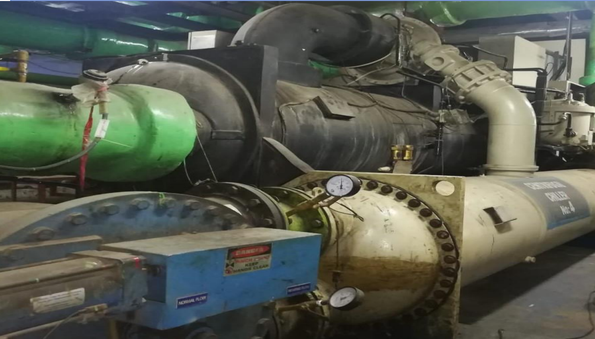
Before Modification (Brush Type Cleaning System in Condenser & Evaporator)
