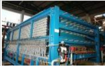
New Udehdehnora Gen.-4 Electrolyser for Caustic Plant 2018-19
