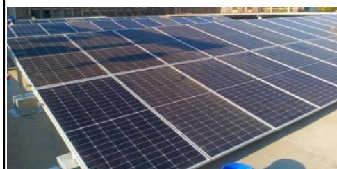
SOLAR PV Power Plant 42 Kw at Main Sub Station.2021
