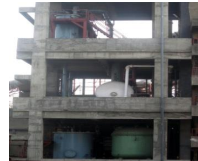
Acid Absorption Crystallizers at T/C Plant 2013-14
