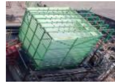
Jet Type Fan less Induced Draft Cooling Tower Jan2017
