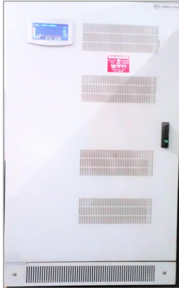
Power Quality Improvement
