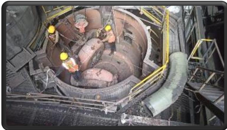
Auxillary power reduction by mill roller replacement
