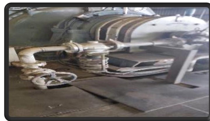
Auxillary power reduction through engineering control
