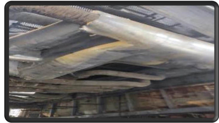
Boiler efficiency improvement by reducing radiation losses
