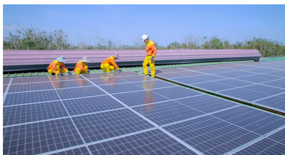
Figure 40: 640kWp Solar Rooftop Plant
