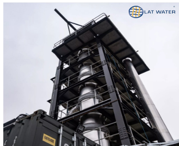
Figure 47: LAT Water installation at Broadpath landfill treating leachate
