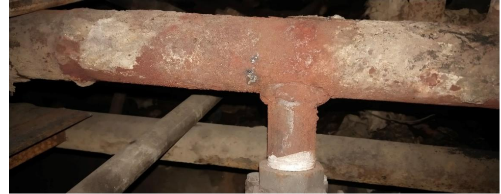
Condensate recovery before
