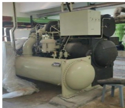
Figure 7: Centrifugal Electrical Chiller
