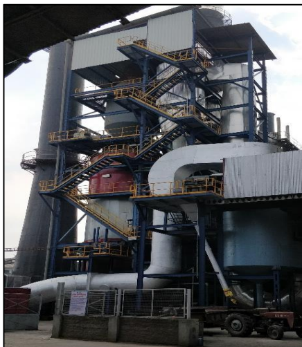
Fig.2. Hybrid Flash Bagasse Dryer integrated to HP Boiler at DSW
