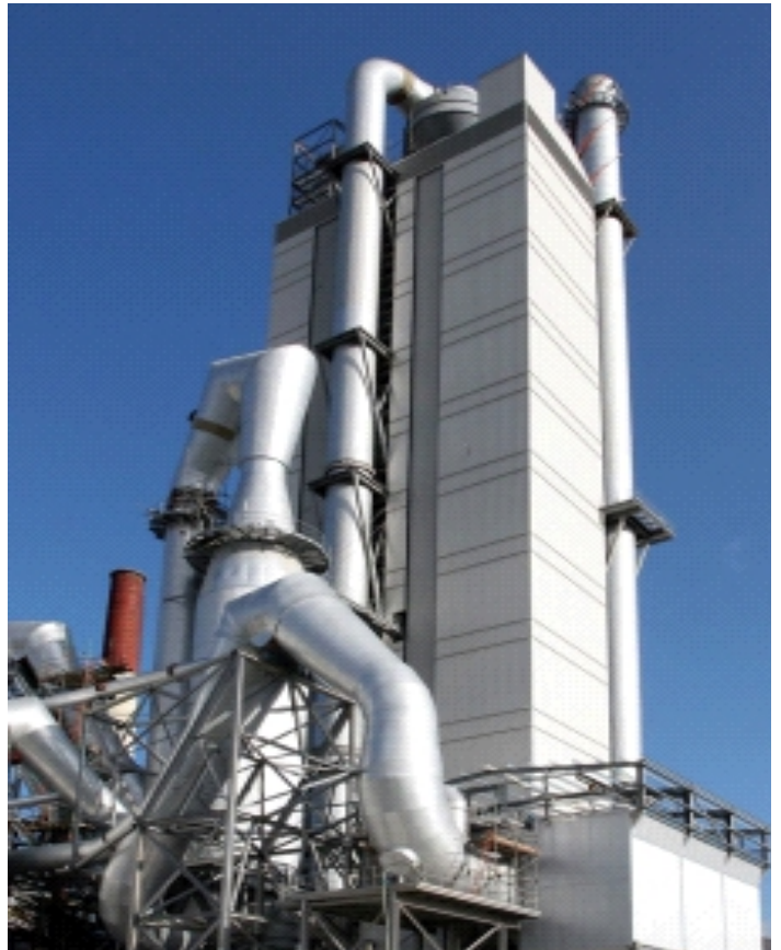
Figure 16: Padeswood Kiln and Cement Plant
