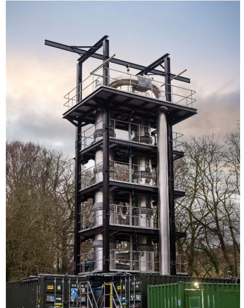
Figure 2: LAT Water installation at Broadpath landfill treating leachate
