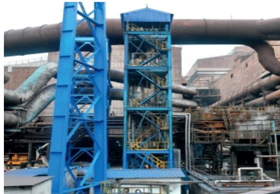
Figure 1: Carbon Clean's CDRMax™ semi-modular technology implemented at Tata Steel, Jamshedpur, India as part of pilot demonstration
