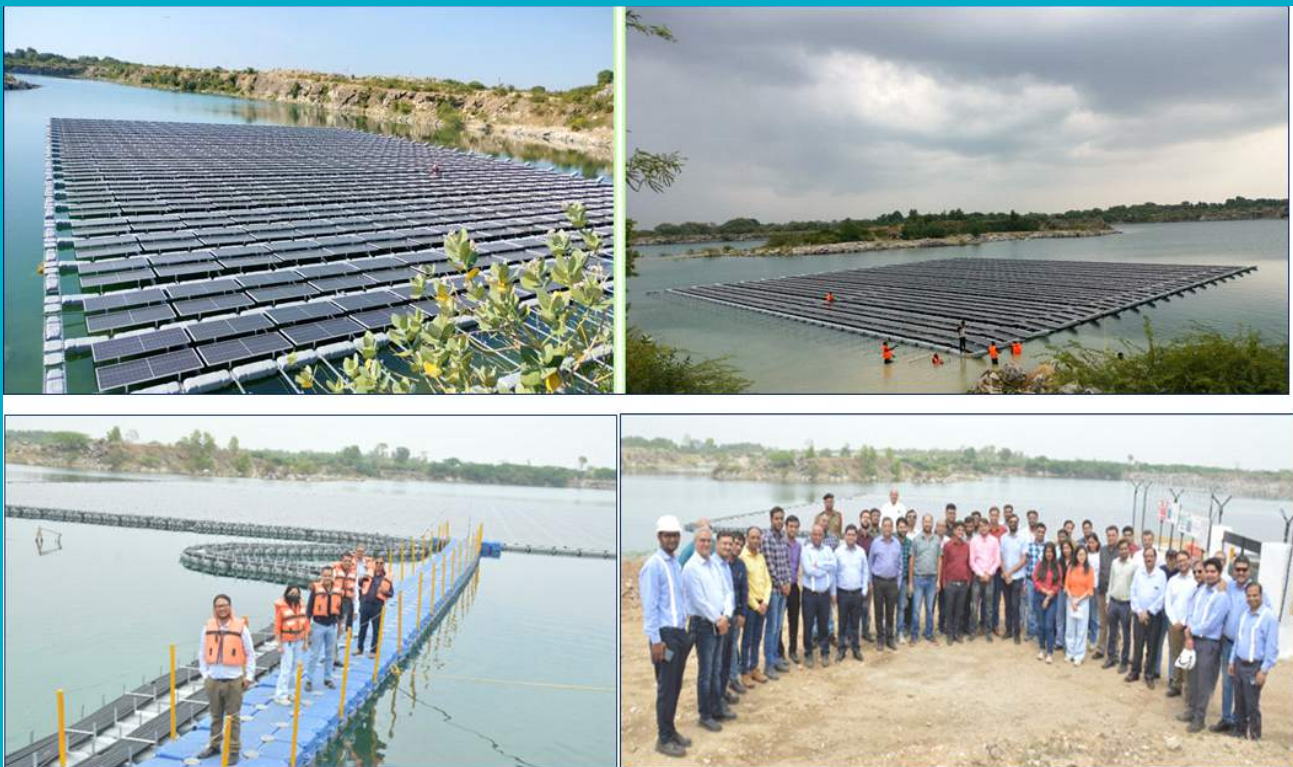
1MW Floating Solar Plant installed at UCWL
