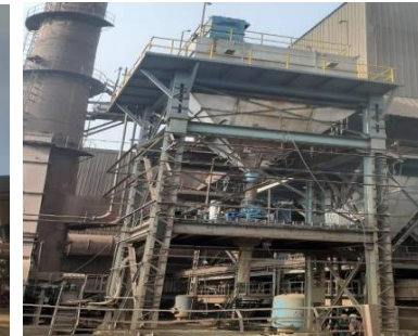
Pneumatic Dust Handling System at SAF # 3, 4 & 5
