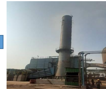
Secondary fume extraction system at SAF # 4 & 5
