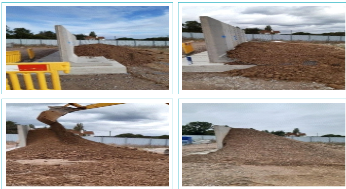
Figure 5: Sequence of backfilling retaining walls with sulphated soil (clockwise from top left)
