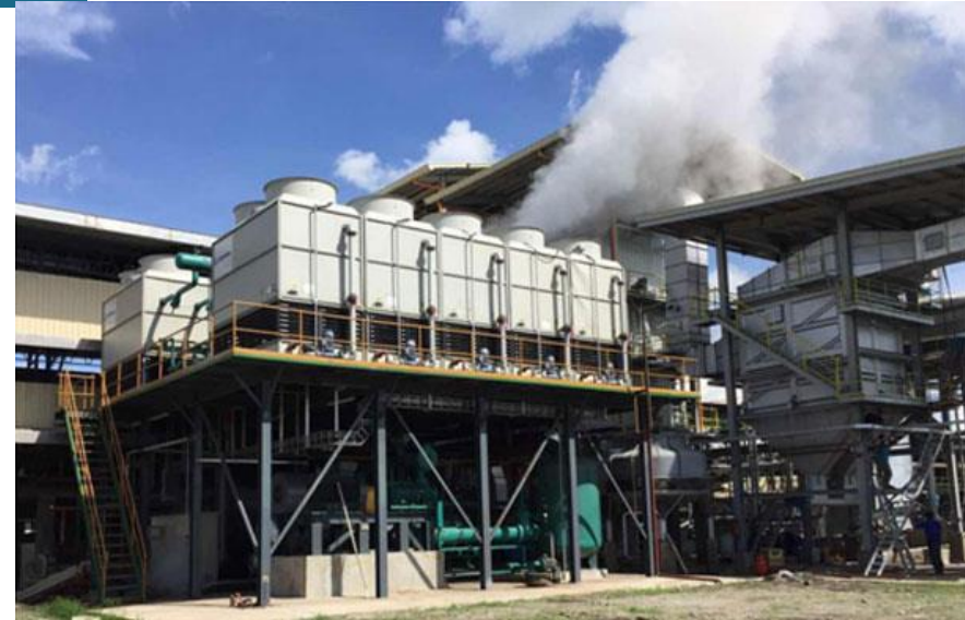
Biomass Power Generation
