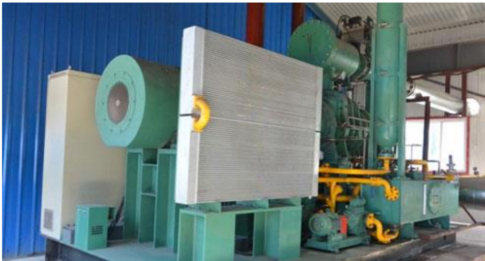
Industry Waste Pressure Power Generation
