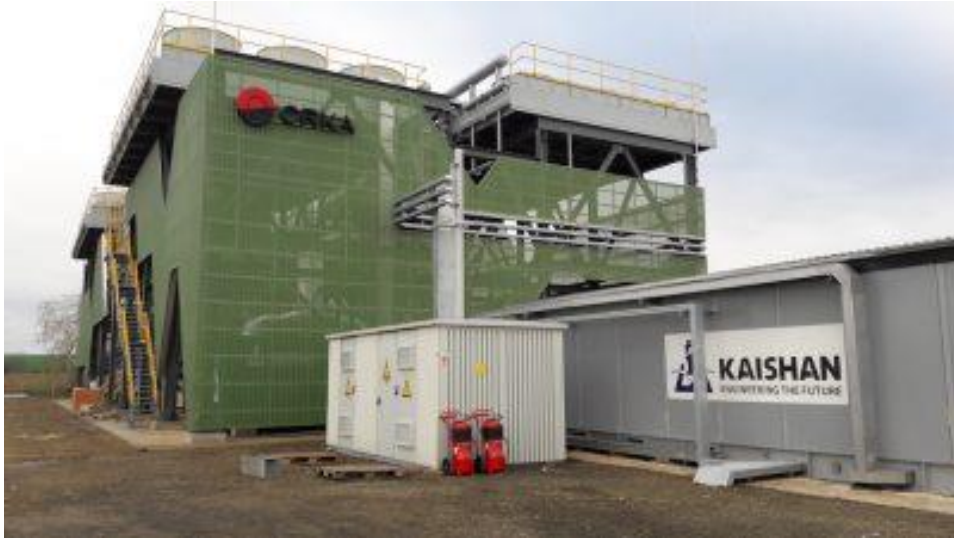
Geothermal Power Generation
