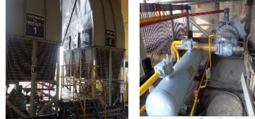
Old System: Refrigerant central AC
