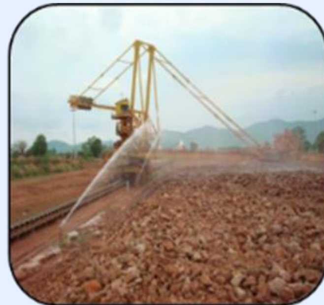
Water sprinklers at bauxite handling
